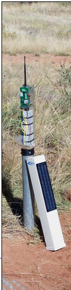
FGRCP LineMarker Test Station
